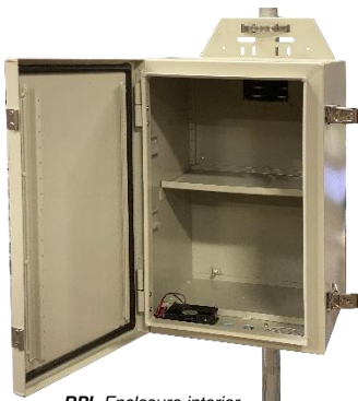
RPL Enclosure interior without batteries or controller
